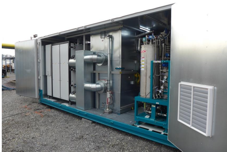
Liquid Organic Hydrogen Carriers (LOHC) applications (the Hydrogenious Technologies StorageBOX) at the United Hydrogen Group (Tennessee, USA). (Photo: Hydrogenious Technologies GmbH)
