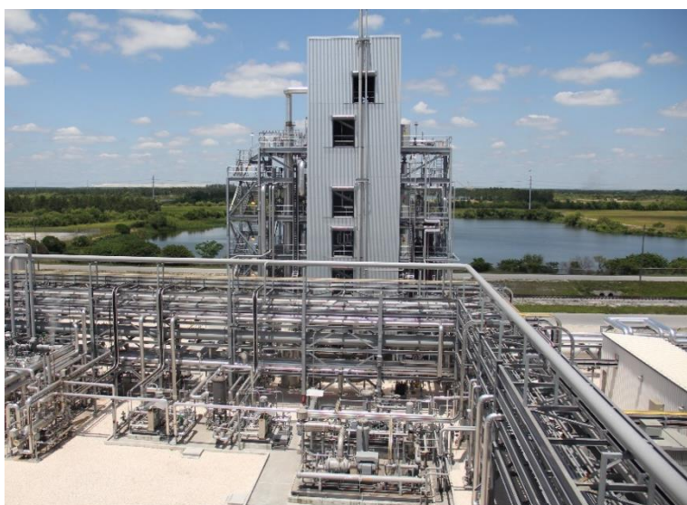
WDP is an advanced technology for producing cleaner energy and chemicals from coal and other high-sulfur feedstocks by enabling sulfur-containing gas streams to be cleaned at elevated temperatures. (Photo: RTI)
